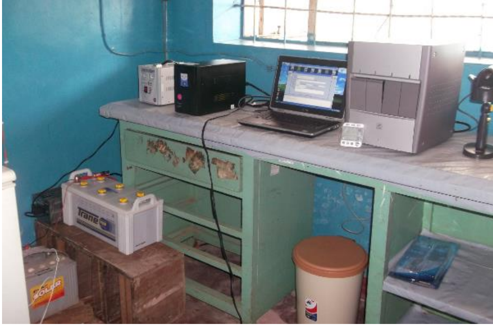
Figure 4.3: Illustration of the electrical installation required for using the GeneXpert in the Shabunda hospital. From the left to the right: battery of the solar panel installation, charger-converter, truck battery, stabilizer, UPS, laptop with internal battery and GeneXpert).
