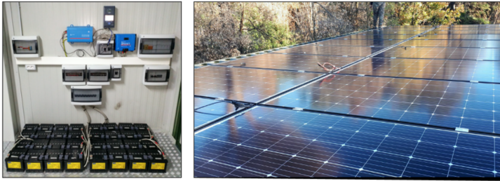
Figure 3.11. | Battery system installed inside the container (left) and solar panels mounted on the roof (right).
