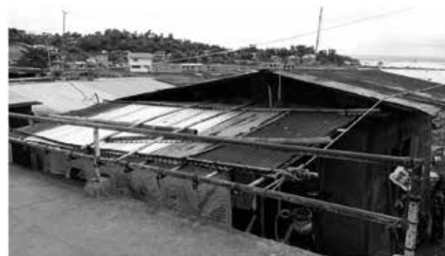
A house on libis is tucked under a road and reinforced with serga . Photo: Angelito Nunag (01 November 2015).
