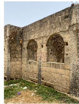
Vacant dwelling, affected by the raising aquifer.
