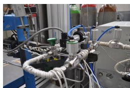
Figure C.12: Vanne manuelle verte pompe secondaire.
