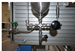
Figure C.9: Vanne verte purge CEM.
