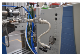
Figure C.25: Vanne entrée GC.
