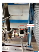
Figure C.13: Vanne manuelle pompe primaire.
