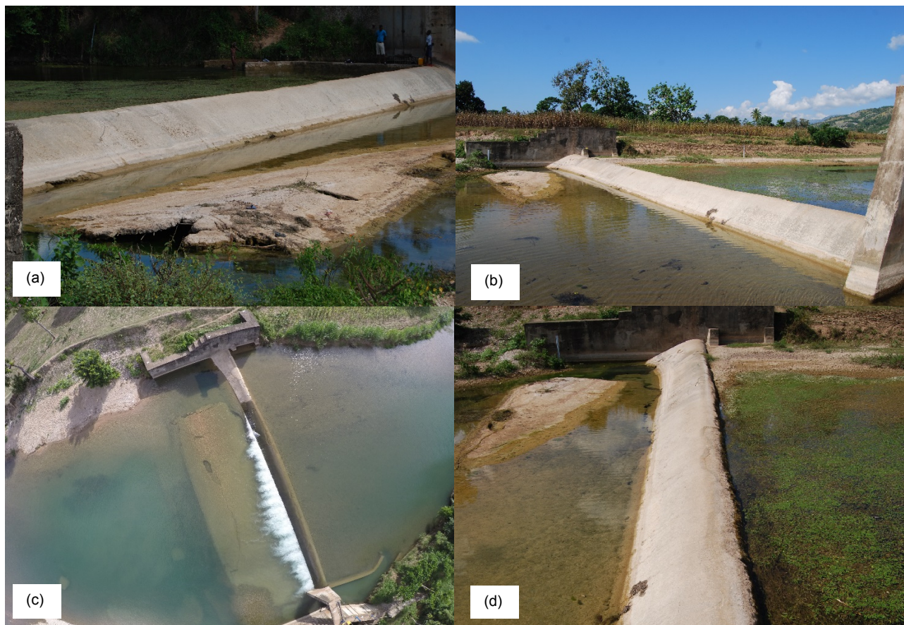
Figure 2. (a) Damaged concrete slab on the downstream face of the weir (b) general view of the Dory weir (c) aerial view of the crest and the downstream slab d) damaged crest and upstream sedimentation.
