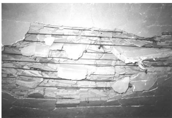
Example of deck decay
