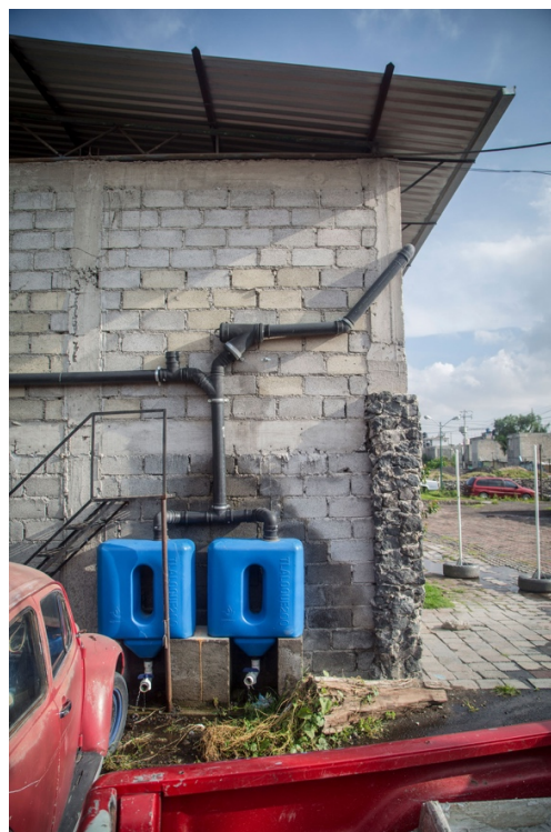
Figure 2 - View of the filtering tanks of the Yuguelito community rainwater treatment plant (© 2015 Isla Urbana with permission).
