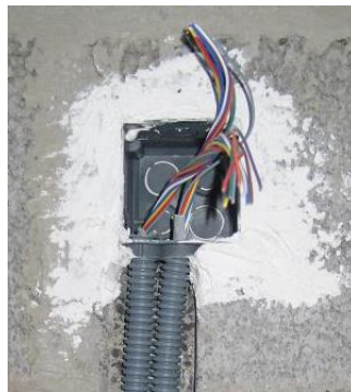
Figure 6: electrical outlet encased in a wall
