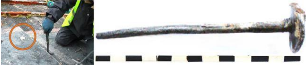
Fig. 80. St. George's Church, Everton, 1813 patent slate system during roof repairs. A 'lead' nail head is circled, left. An extracted 130mm sample, right. Photos Terry Hughes.
