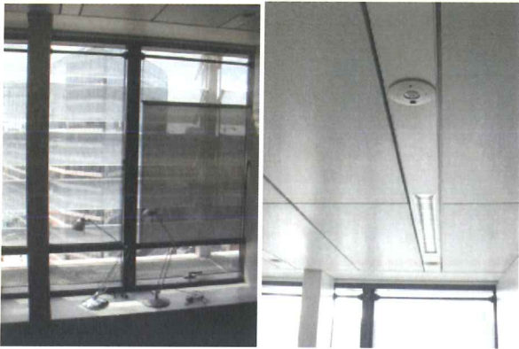
Figure 7: The internal blinds and the automatic sensor system
