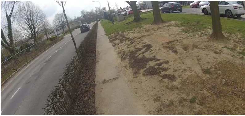
Fig. 4. Participants disliked cycling tracks with cracks and bumps.
