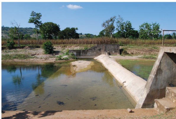
Fig. 6 : Damaged Dory weir.
