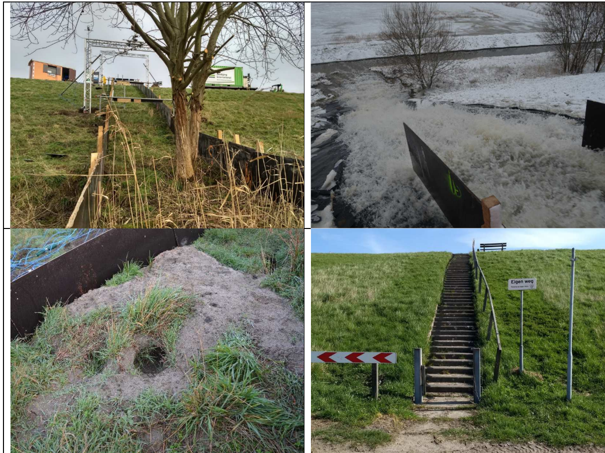
Figure 7. Top left: Test section with a tree at the bottom end of the landside slope, prior to overflow test, picture taken by Stephan Rikkert on February 16, 2021. Top right: Overflow test on an emergency repair measure: damaged landside slope was covered with EPDM foil, picture taken by André Koelewijn on February 7, 2021. Bottom left: Prepared test section with fox holes present at the landside slope, picture taken by André Koelewijn on November 23, 2020. Bottom right: Test location with stairs, to study soil-structure interaction, prior to overflow test, picture taken by Stephan Rikkert on March 30, 2021.
