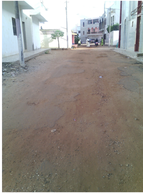
Figure 10.15: Dirt Road in Soprim 1
