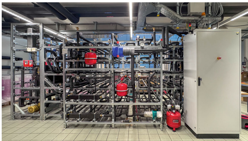
Fig. 3 ROADMAP project 6GDHCN experimental facility
