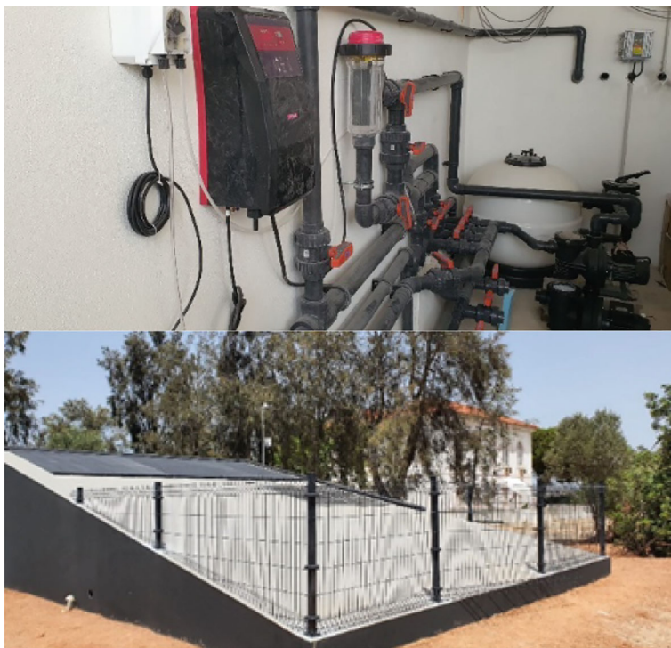
Fig. 6 Machine room with hydraulic circuits
