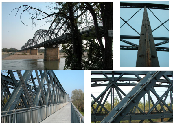
Figure 1. Truss members deformed by rust swelling.
