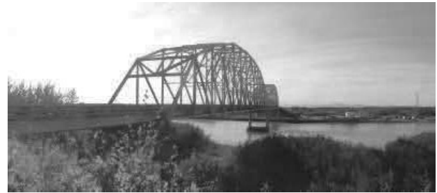
Figure 7. Picture of the bridge structure and the pier in the riverbed (photo credit: Don Moe, http://donmoe.com/blog/2016/01/15/fairbanks-ak-to-denali-highway/ ).
