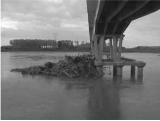
Figure 1. Clogging phenomenon on a bridge over the Po River, Pieve Porto Morone, Italy (Malerba, et al. 2013).
