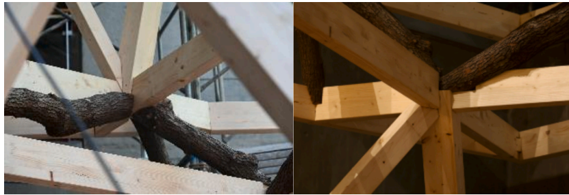
Fig. 17. Detailed views of Joint 16 and Joint 20.
