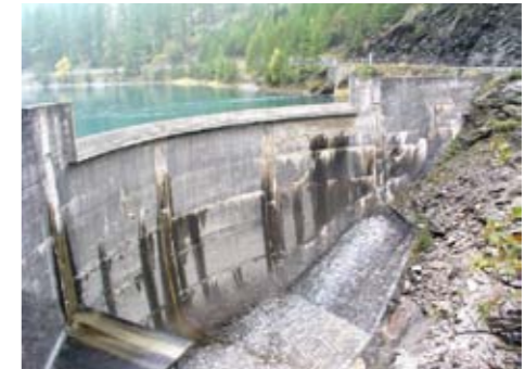
Figure 1: dam affected by ASR (Isee, Switzerland)
