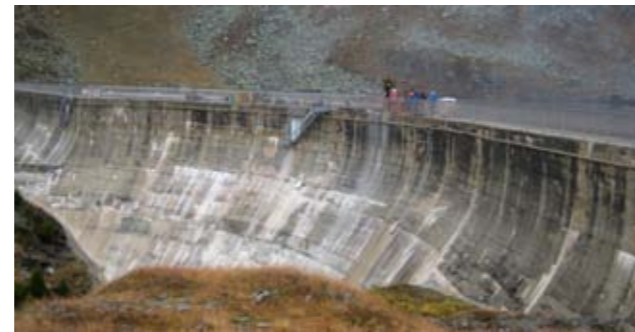
Figure 1: ASR affected dam in the Swiss Alps
